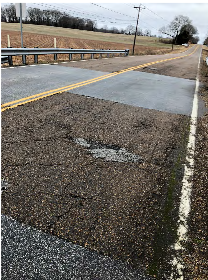
Spalling and Cracking along Surface
