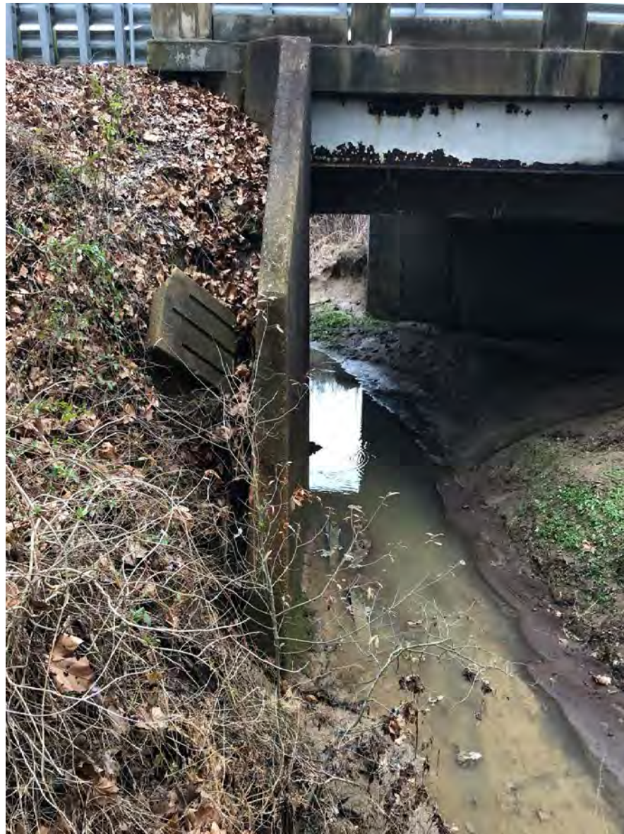
Washout and Vegetation on West Abutment at Inlet
