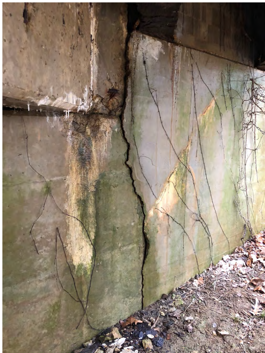
West Abutment Decay and Cracking
