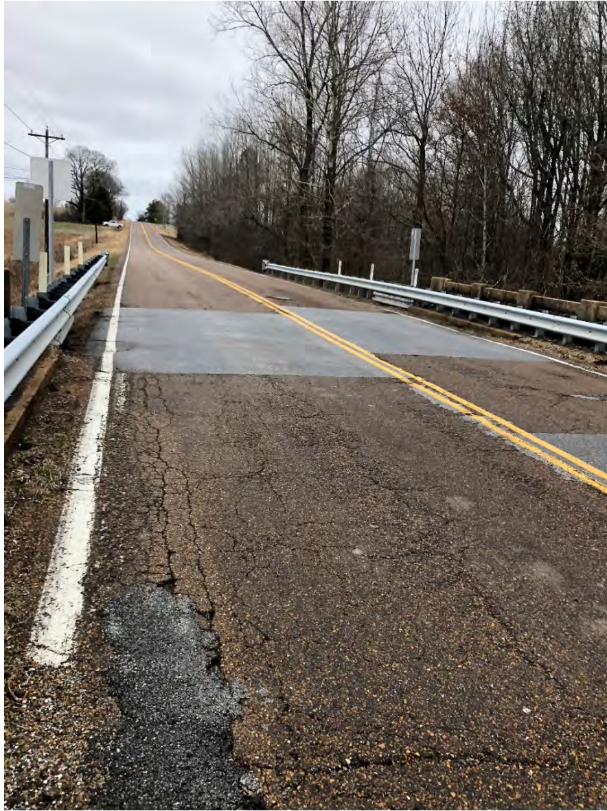
Pavement Cracking and Spalling along Surface from West Abutment
